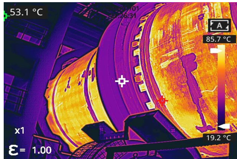
Rotary Kiln Defect Monitoring
